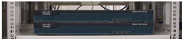
Access Routers (Dual)
