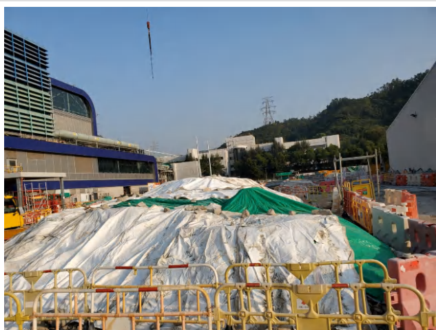
Cover stockpile of soil material to prevent generation of fugitive dust and surface run off
