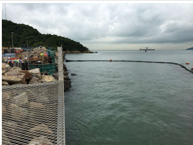
Use of silt curtain as precautionary measure to prevent construction works near the sea from causing suspended sediment impacts to marine environment
